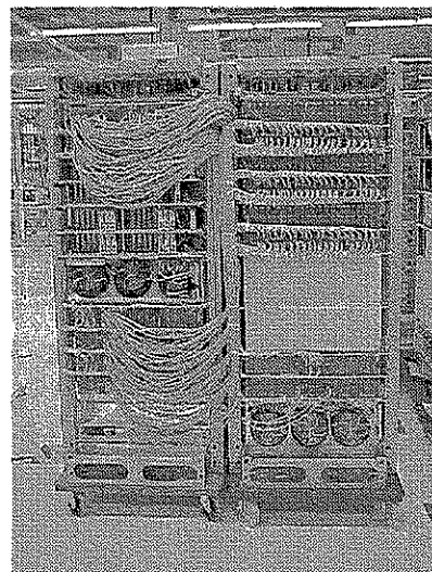
5ESS® Switch, rear view
